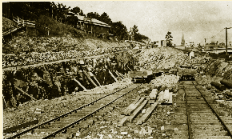
c1918, Excavation of land for extensions to Roma Street Goods Yards. (JOL 37398)
